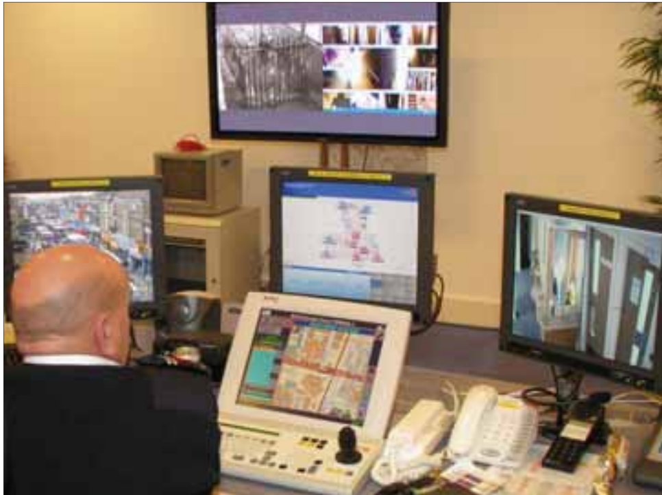
CNL’s IP Security Centre will control all of Enfield’s security systems
